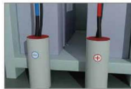
sealing of pipes where cables running through
